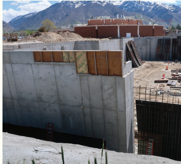
ABOVE: PHASE ONE CONSTRUCTION SHOWING THE 35-FOOT ELEVATION DROP BETWEEN THE OLD AND NEW STRUCTURES.
